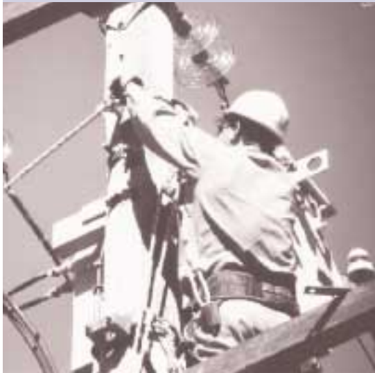
Photo courtesy of Western Power
