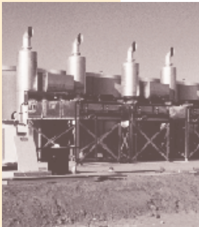
Photo courtesy of Western Power
