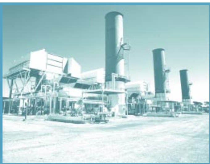
Parkeston power station now accesses the grid.
