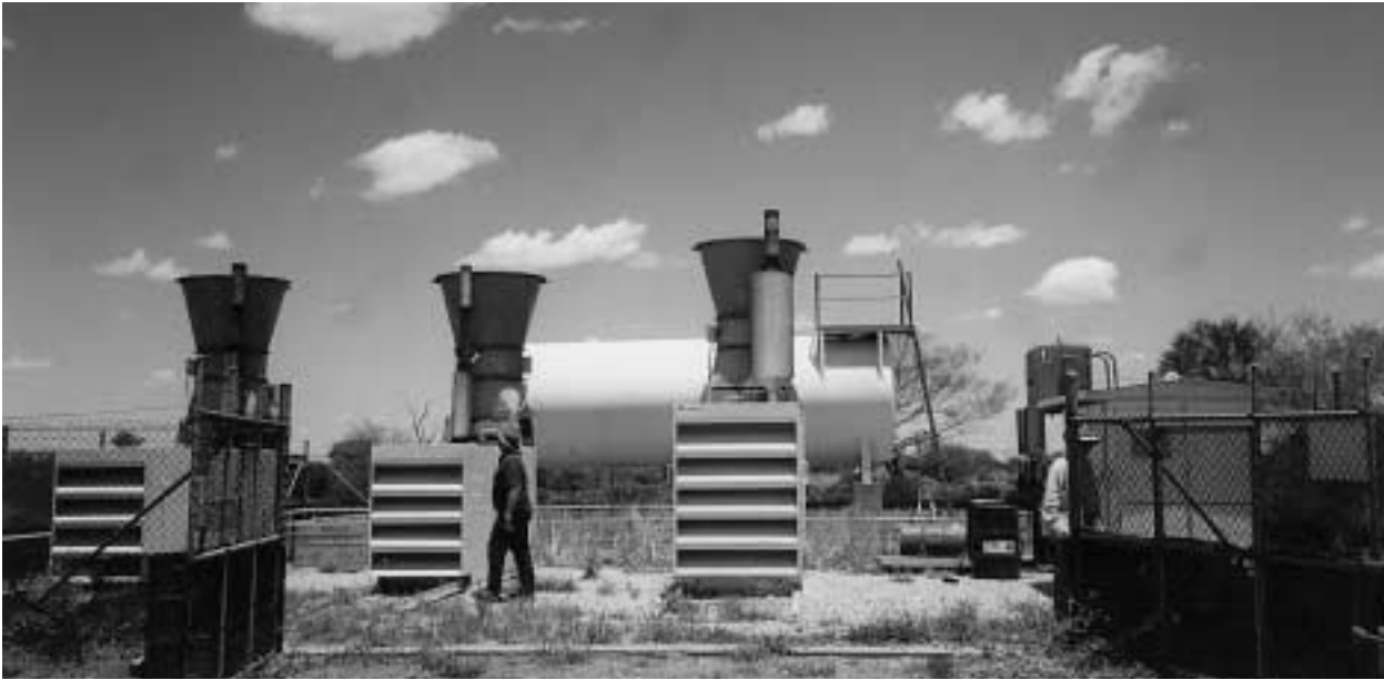
Outdated diesel power units will be replaced as part of the remote community pilot project in the Kimberley.
