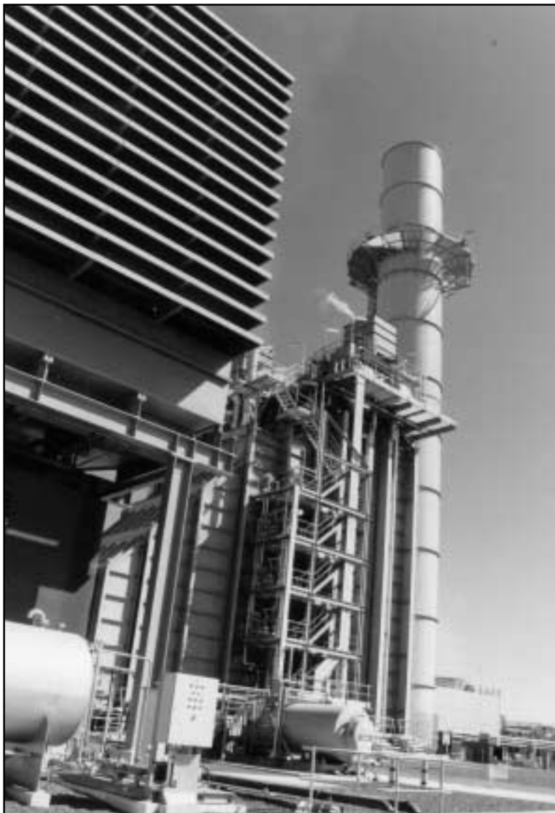
The cogeneration facility, one of the biggest of its kind in Australia, supplies electricity and steam to Worsley alumina refinery and electricity to Western Power’s South West interconnected system.
